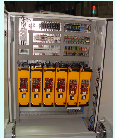
Main Electrical Cabinet
